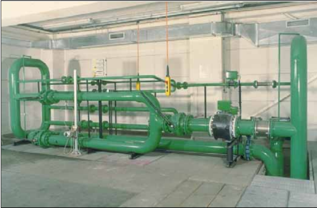
Fig. 4: Water calibration test stand for pipe sizes DN 15 (1/2") to DN 300 (12"). Volumetric flow: 0 to 360 m 3 /h (1600 GPM). Temperature: 15 bis 25 °C. Druck: 0.2 – 1.,0 bar.
